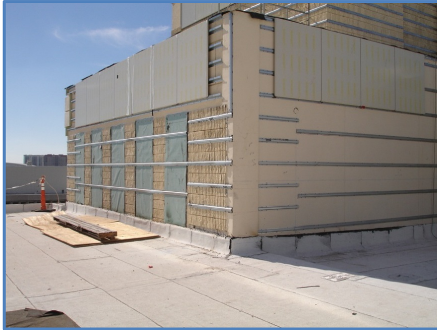
Figure 1: North Criminal Courthouse Annex Re-roof and Wall cladding is one of current County renovation projects.
