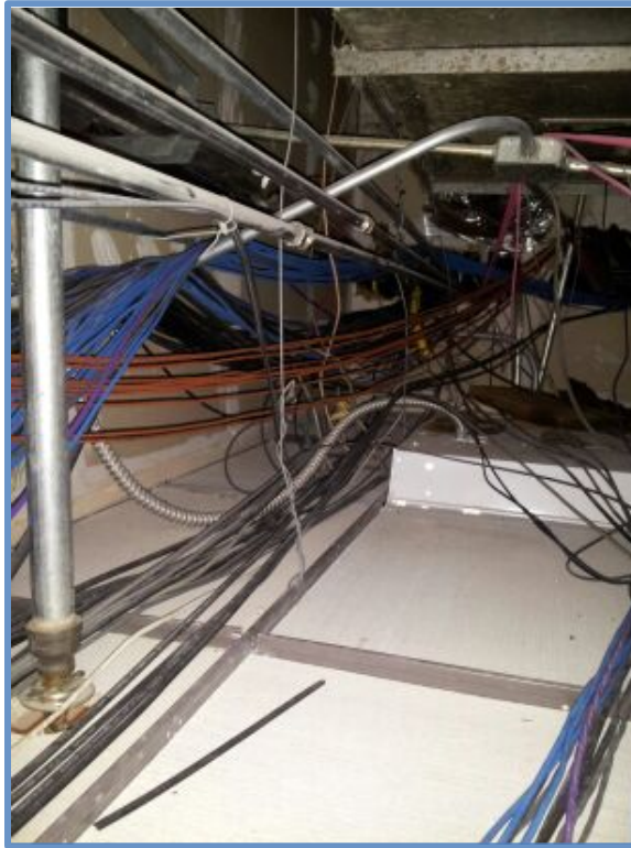
Figure 12: Retrofitting the Criminal Courthouse Complex, built in 1962, leaves little space for new technology due to previous retrofits.
